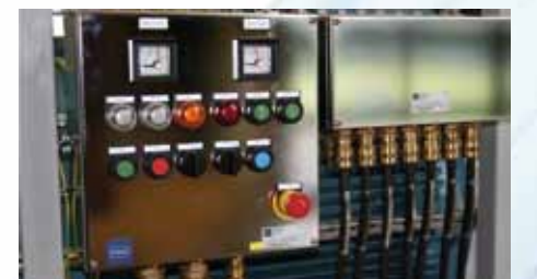
Above: Operation by Local control panel
